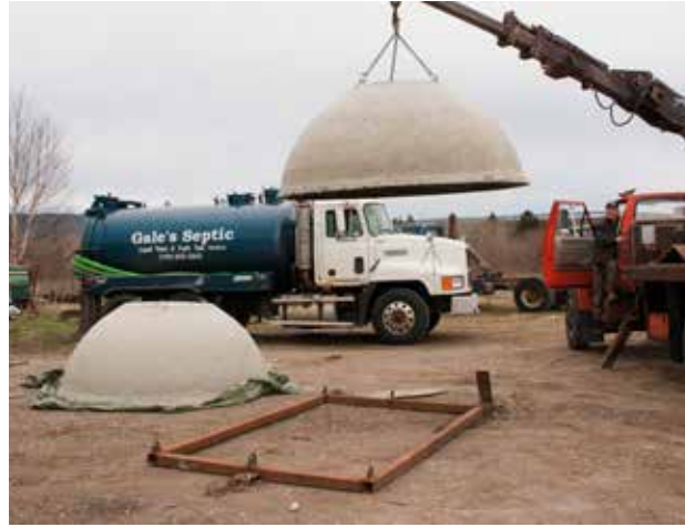
Left: Gerard Gale works the boom truck, moving a freshly made tank half at the Gale's Septic yard.
