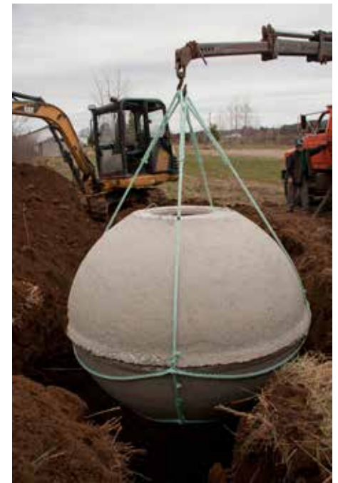
Below: Gerard Gale stands by the boom truck while a new Turtle Tank is lowered into the ground.
